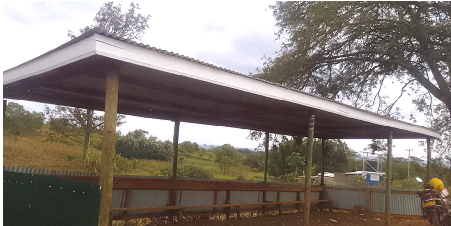
Photos 7: Ongoing construction of a boda boda shade for double GM SHG in Mutithi
