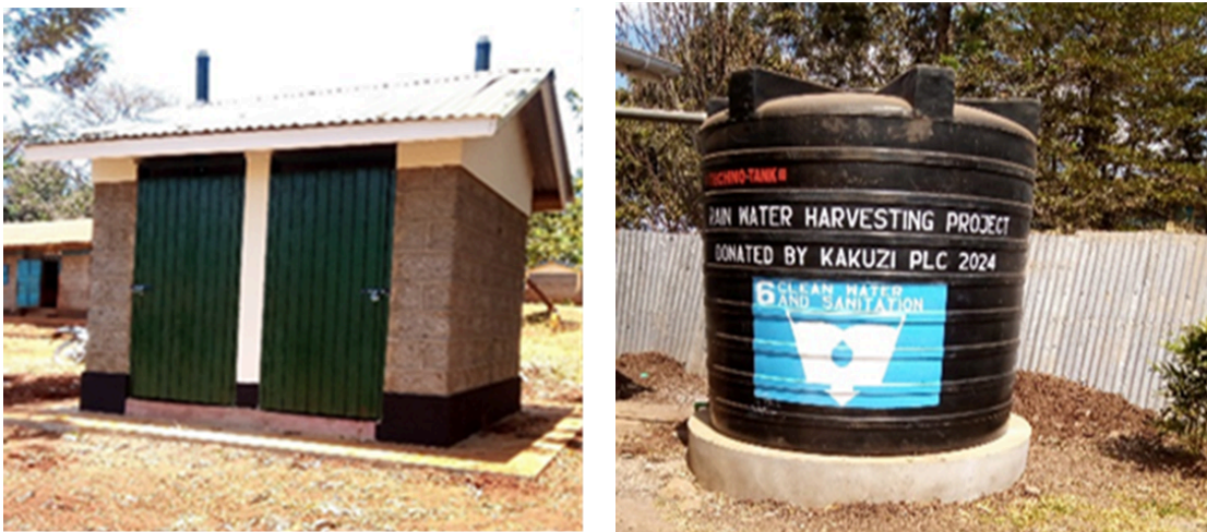
Photo 6: Complete rainwater harvesting system& a 4- door sanitation facility at Gituamba health facility & Githanji Primary School
