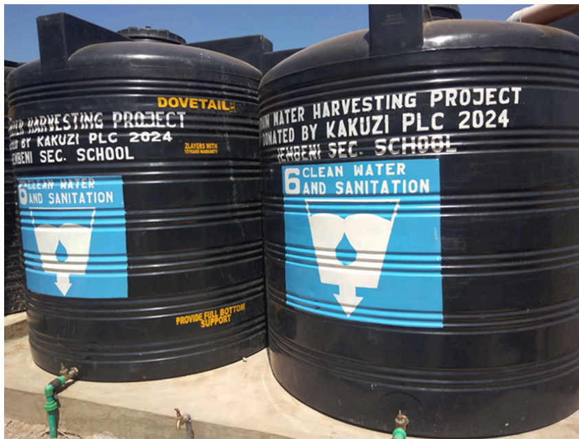
Photos 5: Complete rain water harvesting system at lembeni Secondary School
